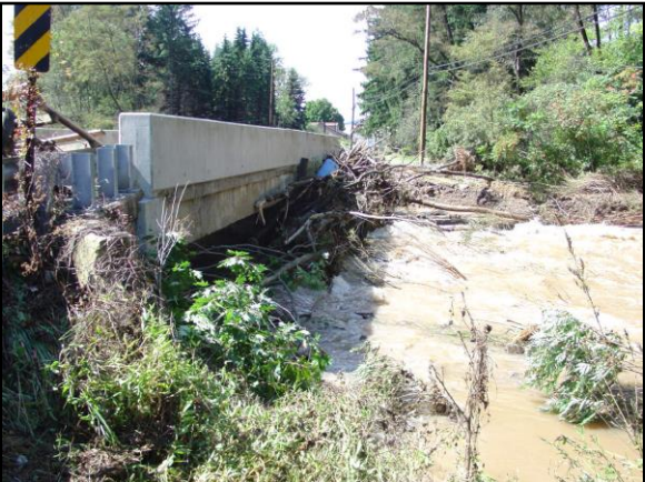
Severe debris buildup of tree branches, caught against the bridge blocking more than 25% of the span opening
