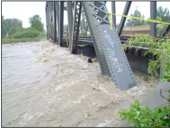
Pressure flow – water is flowing against or the bridge superstructure. Water levels may continue to rise and flow over the bridge; this is called “overtopping”.
