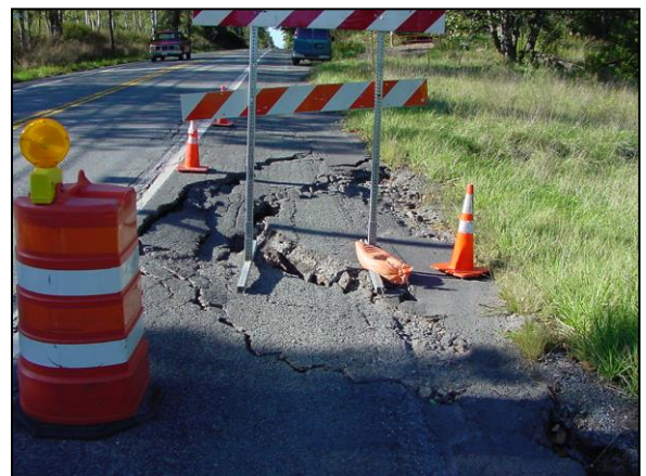
Settlement damage effect on the roadway due to scour underneath the bridge abutment in the picture to the left
