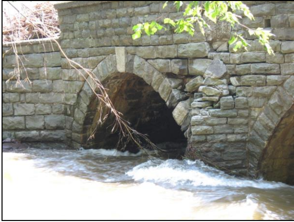
Settlement damage in the stone masonry pier and some collapsing in the arch
