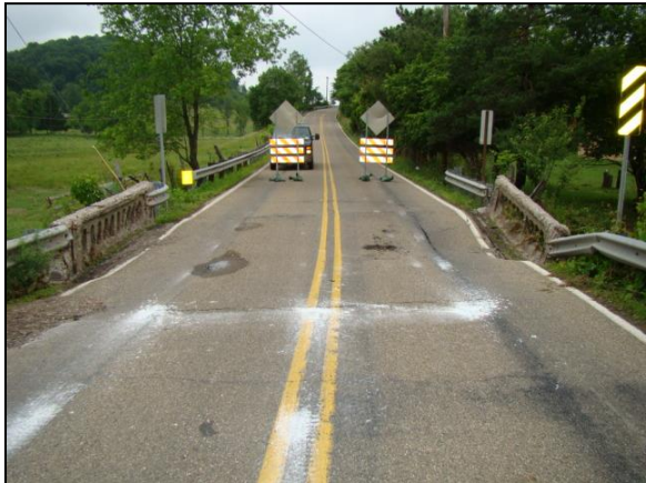
Settlement damage in the roadway due to settlement and tilt of the bridge abutment in the picture to the right
