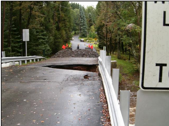
Extreme settlement damage in the roadway, causing a hole in the roadway behind the bridge abutments
